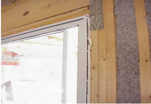
Figure 7. Good insulation detail of blown cellulose installation and foam insulation around window frame.
