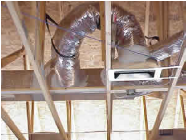
Figure 6. Mastic sealed attic supply duct and plenum.
