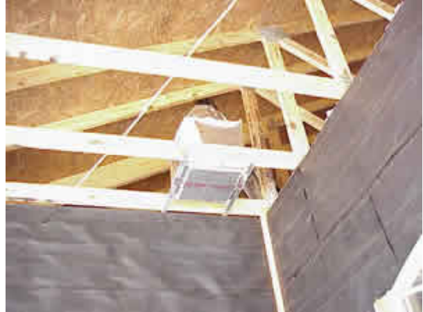
Figure 8. Outside air provides controlled, filtered fresh air while maintaining household at positive pressure with reference to outside pressure.
